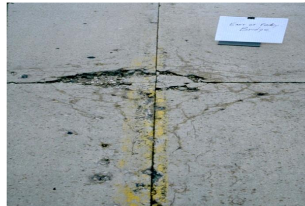
Pavement damage from D-cracking
