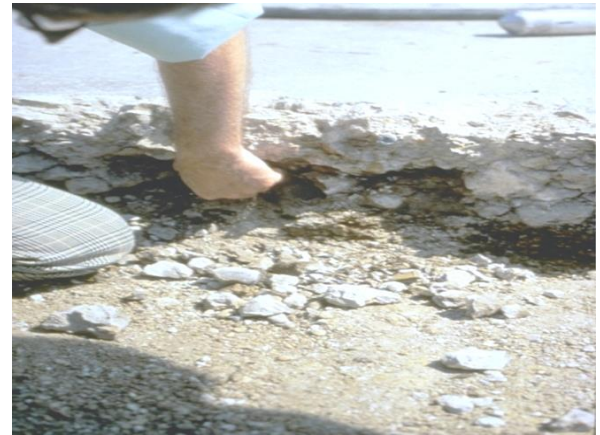
Pavement damage from D-cracking
